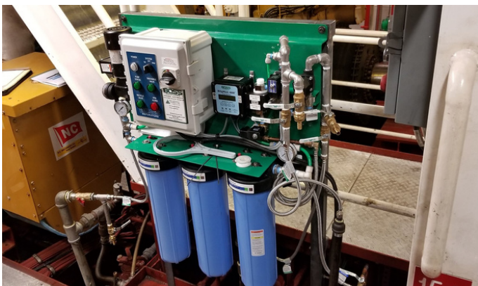
WATER TREATMENT & SEPARATORS
